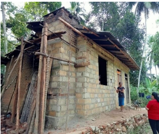
Damaged roof and wall undergoing repair and replacement – Rathnapura District (Photo: SLRCS)
